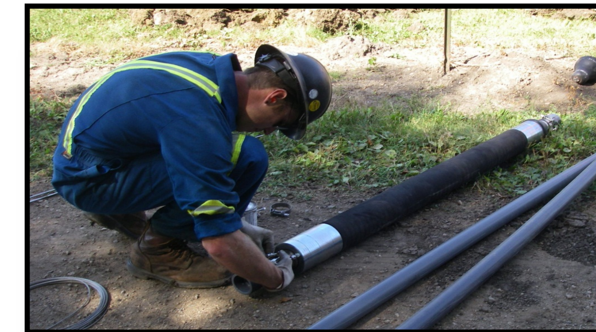
(Photo 2: View of the inflatable packer being assembled to the horizontal well.)
