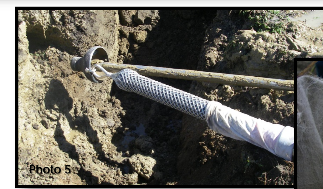
(Photo 5 and Photo 6: The assembled carrier casing well being installed into the borehole. Note the filter sock covering on both the outer (Photo 5) and inner (Photo 6) wells.)
