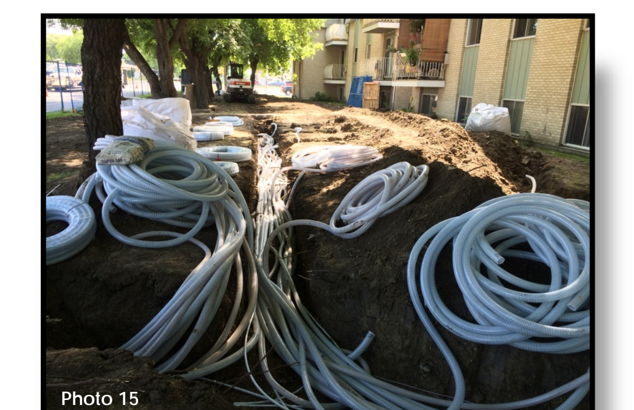
(Photo 15: View facing east of the north side of the apartment building. Approximately 2,500 m of dedicated header line was used during the installation.)
