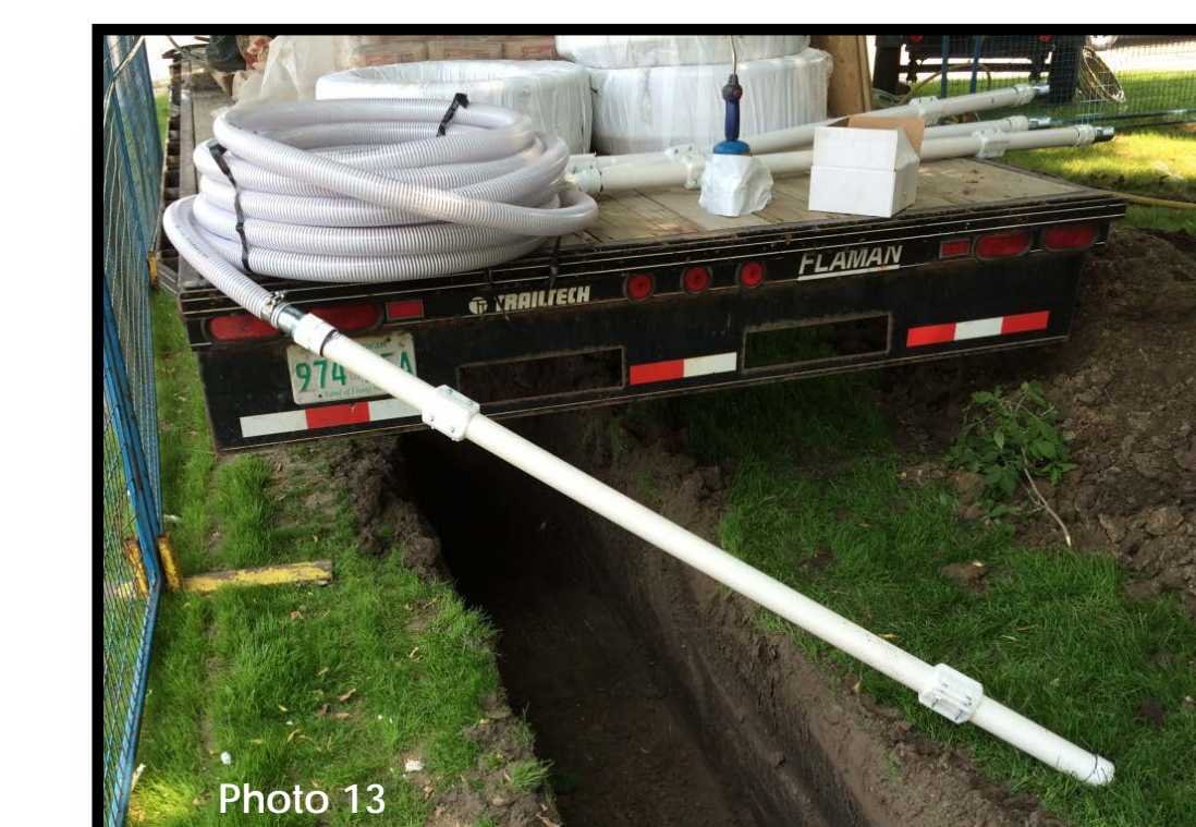
(Photo 13 and Photo 14: View of unique vertical recovery well design. Note the well screen is attached directly to the header line without elbows or connectors, thus reducing vacuum friction loss. Centralizers were also attached for proper positioning.)
