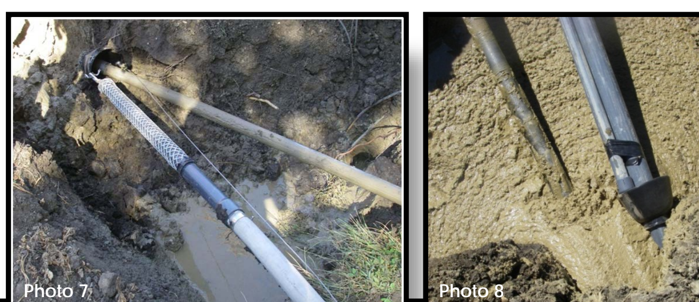
(Photo 7 and Photo 8: View showing the standard PVC well concept being installed into the borehole. Note the well is attached to the specialty tooling adaptor using a cable grip.)
