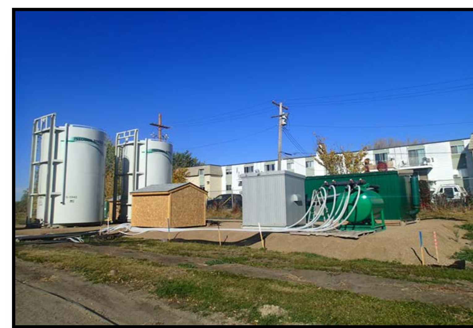
(Photo 1: Facing northwest, view of the remediation system components. Note the apartment building in the background.)
